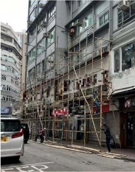
Figure 9: Inadequate safety equipment for workers on the bamboo scaffold (Taken by our staff in January 2024)
