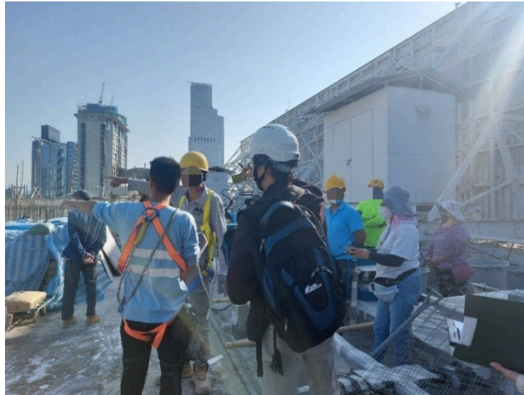
Figure 5: Workers not wearing safety helmets, including the foreman (far left) (Photograph taken by our staff in January 2024)
