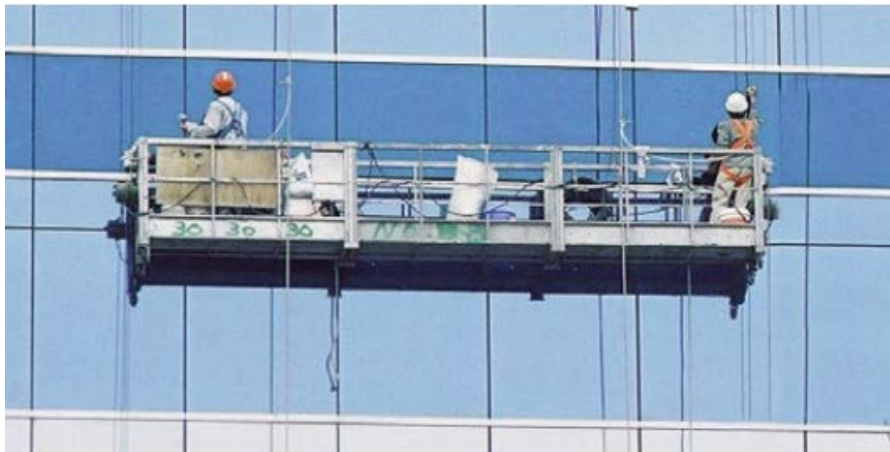
Figure 2: Suspended working platform (Taken from LD's website)
